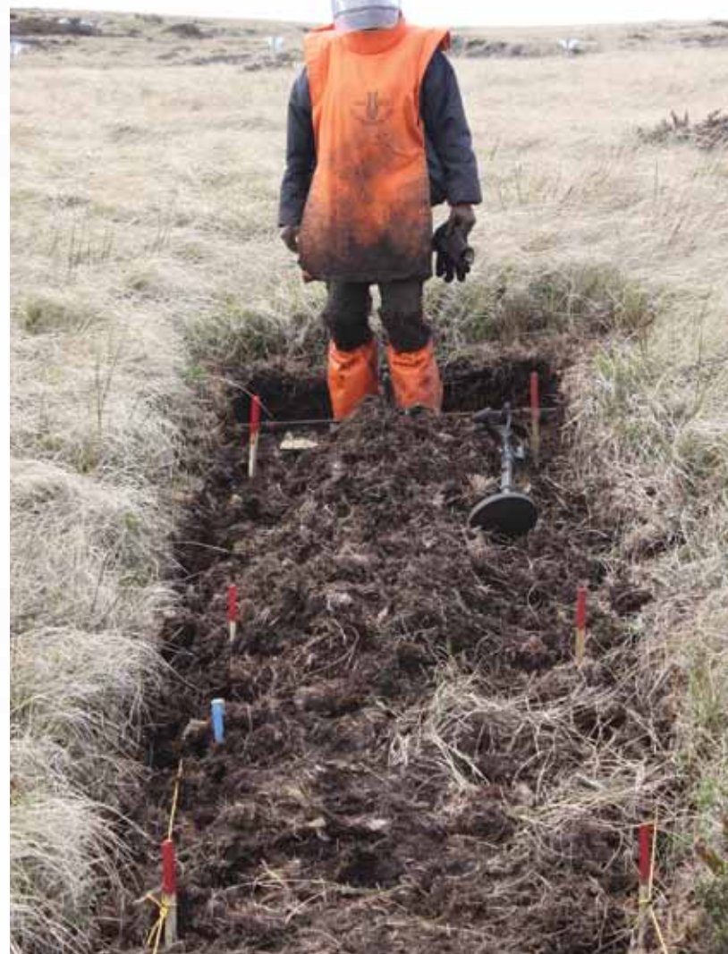
Fully excavating the access lanes on Sapper Hill before the first P4Bs were encountered. PHOTO COURTESY OF GUY MAROT, DPO TECHNICAL ADVISER
