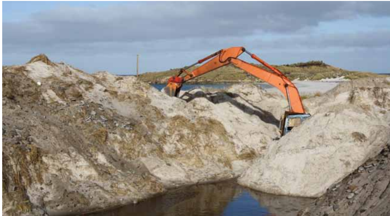
Armored excavator searching for the SB81 mines at the 1982 profile within the Surf Bay Sand Dunes. PHOTO COURTESY OF THE AUTHOR
