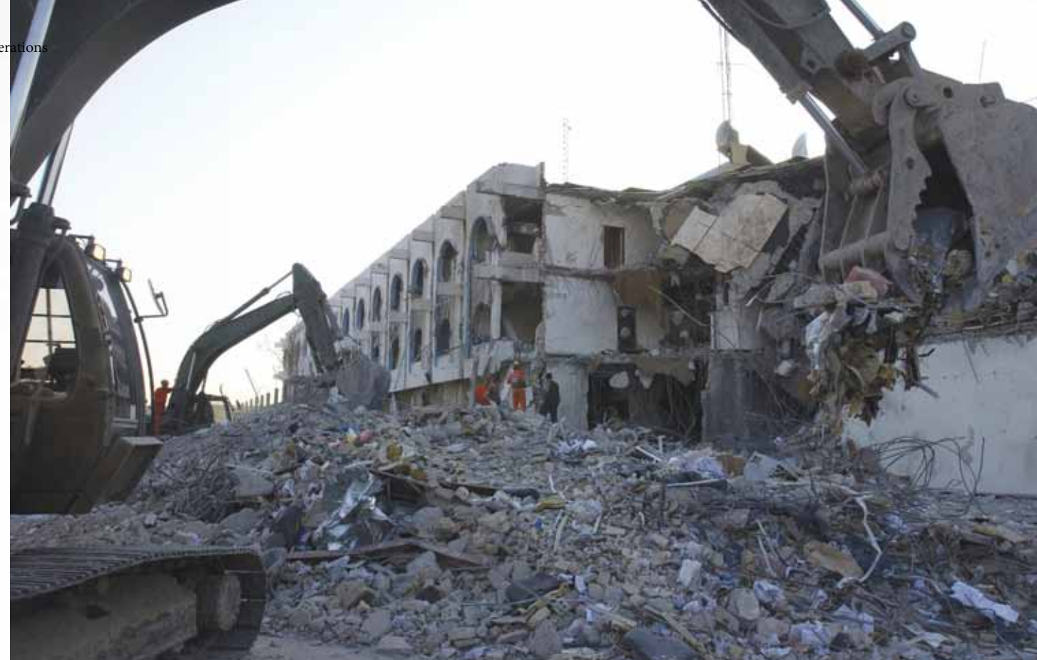
U.S. Army soldiers assigned to the 203 rd Combat Engineer Battalion of the Missouri Army National Guard use a tracked excavator to remove tons of rubble and debris as rescue workers search for victims at the United Nations Office of the Humanitarian Coordinator building in Baghdad, Iraq, after a truck bomb destroyed much of the building on 19 August 2003.
