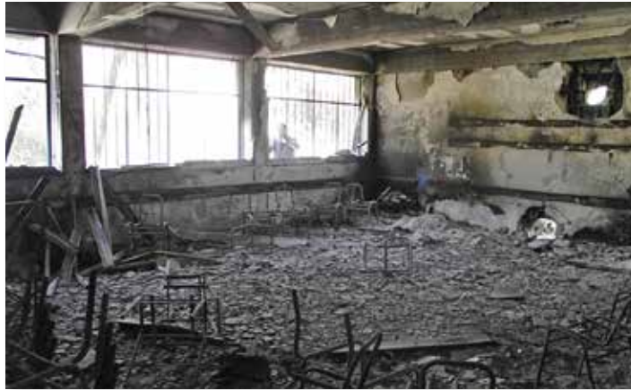
UNRWA classroom in Biet Hanoon.
