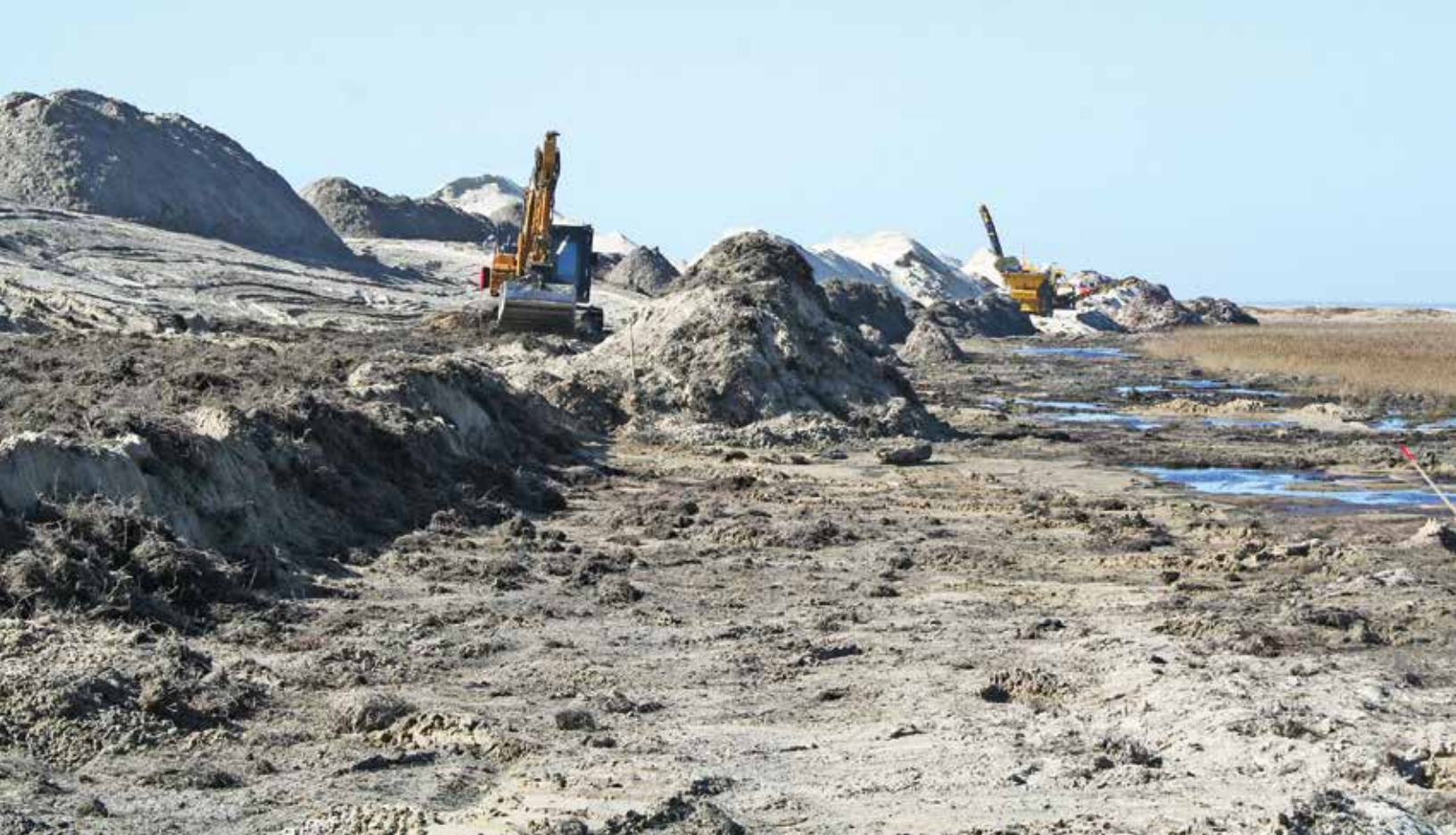
This picture was taken during the reconstruction of the dunes after the mines had been cleared. Without the environmental constraints and rehabilitation of the area it would have had limited value for the wildlife and population following mine clearance.
