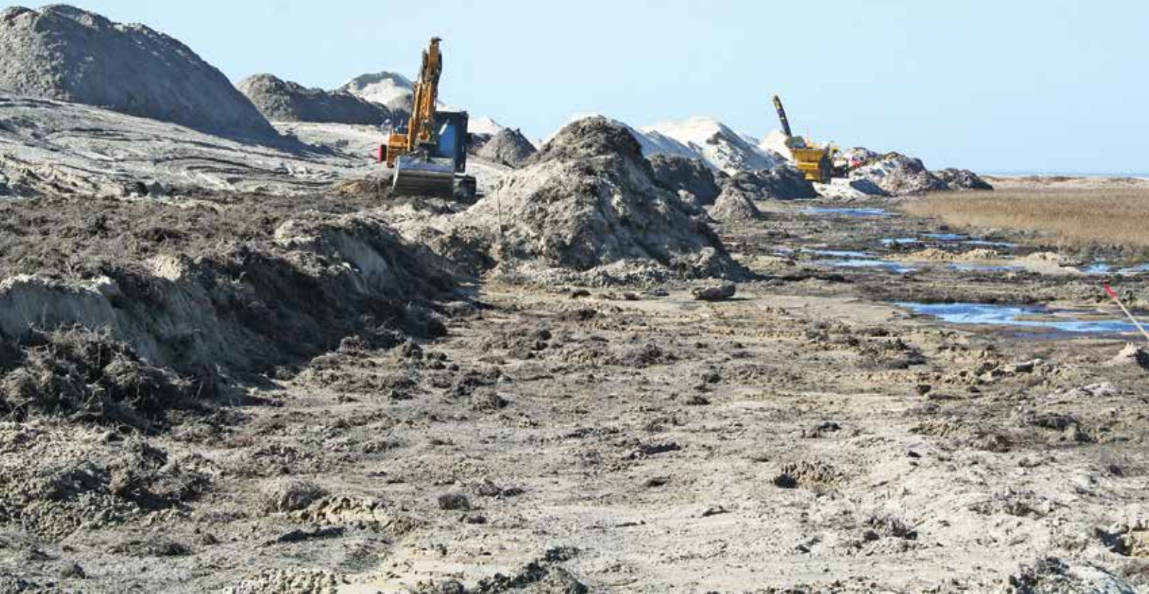
This picture was taken during the reconstruction of the dunes after the mines had been cleared. Without the environmental constraints and rehabilitation of the area it would have had limited value for the wildlife and population following mine clearance.
