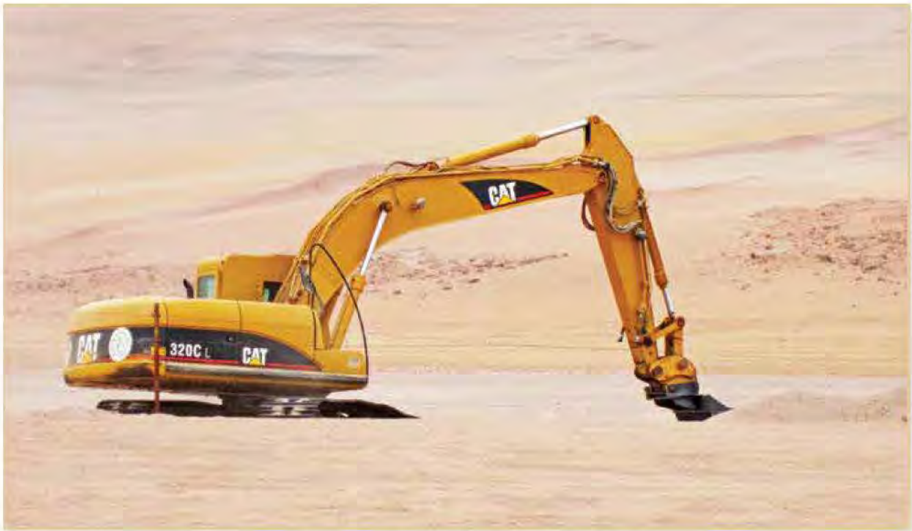
The Multi-Tooled Excavator with an armor protected cab works deep in a dry creek bed to clear anti-tank and anti-personnel mines. Photo courtesy C. Wanner, U.S. Dept. of Defense, Humanitarian Demining Research and Development Program.
