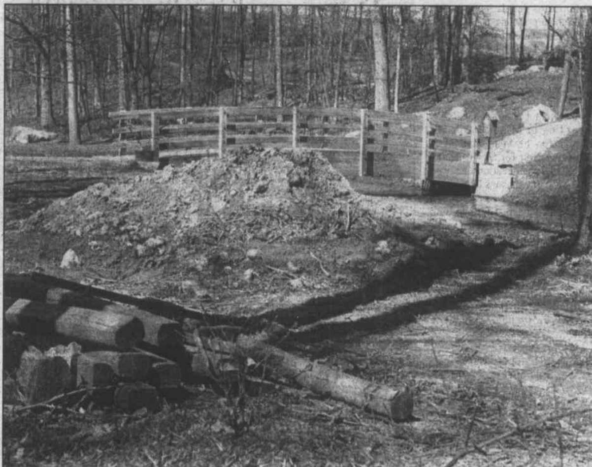
A pile of dirt and pieces of wood show signs of spring cleanup in progress at the Arboretum, Saturday afternoon. Repairs are a necessary chore after the damage this winter's flood inflicted.
