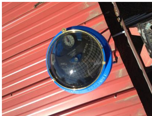
Image 5. Photograph of the Solar Pathfinder on the Workhouse Roof.
