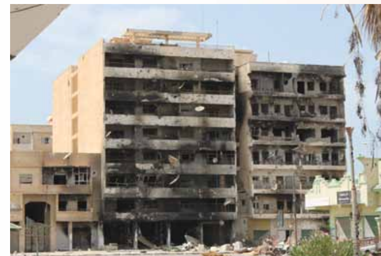
An area showing more moderate damage. Much of the damage to this building is from fires rather than from the blast or fragmentation effects of UXO. A small number of UXO items were found in the buildings pictured.
