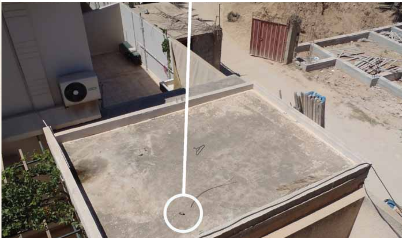
Top left. DCA teams working around "Severe" damaged buildings. Top right. An MRE poster provided by Handicap International. Center and bottom. This cluster munition was reported to DCA by a resident who could see it on the garage of his neighbor's house. It would have been missed by BAC teams who would not have been granted access to the house, and it would not have been spotted by the householder as there is no view over the garage from the house.
