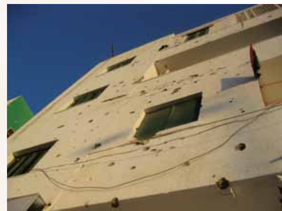
An example of low amounts of battle damage. No items of UXO were found around this building.
