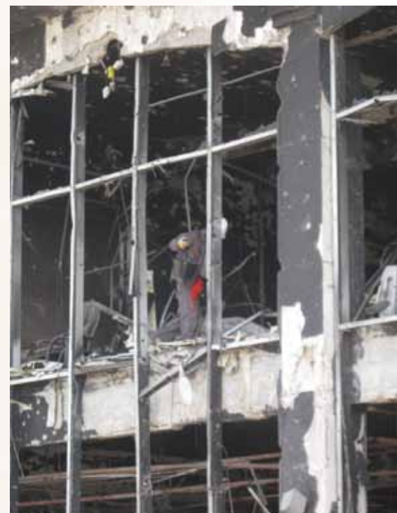
A DCA searcher checks severe damage to a building. The building includes a great deal of blast damage and collapse in some areas. An item of UXO was found on the roof of this building.
