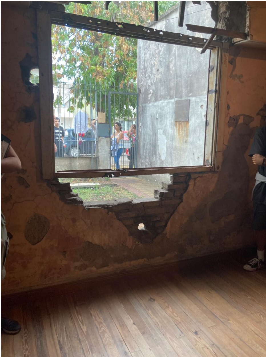
Figure 8. View from inside the house, looking through the wall that was almost entirely destroyed in the attack. The tour guide mentioned how the police intentionally caused a lot of damage to this wall, as it faced the street and was the most visible. See http://asociacionanahi.org.ar/ .
