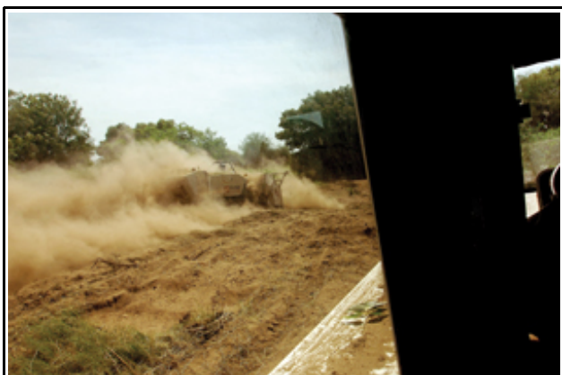
Engineers from ArmorGroup use MineWolf demining machines to clear AP landmines under a program coordinated by the UNMAO in consultation with the Government of Southern Sudan and other national and international actors. Approximately 2,000 AP mines
