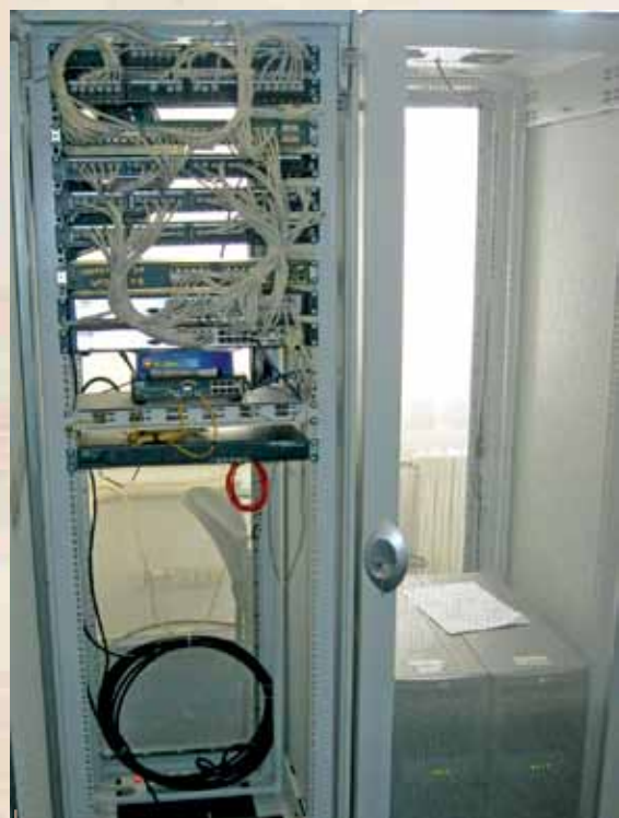
A network rack containing equipment. All photos and graphics courtesy of the author.
