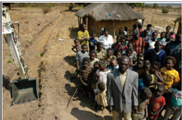
Jermias Matuca, Deputy Chief of Luangrico village in Angola's Moxico province, stands by with his community as a MAG excavator finishes an irrigation canal, having cleared the land of mines.
