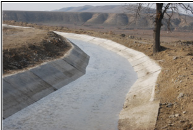
A repaired aqueduct in Azerbaijan supported by ANAMA. All photos courtesy of Charles Downs
