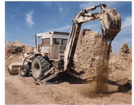
Figure 1: Backhoe used in Khandahar, Afghanistan for excavating residential areas. Dirt spread by the bucket is inspected visually for mines and small UXO devices. The operator is shielded by steel plate around the cab, and 25mm thick polycarbonate windows. A second operator watches from a nearby vantage point and alerts the operator by radio.
