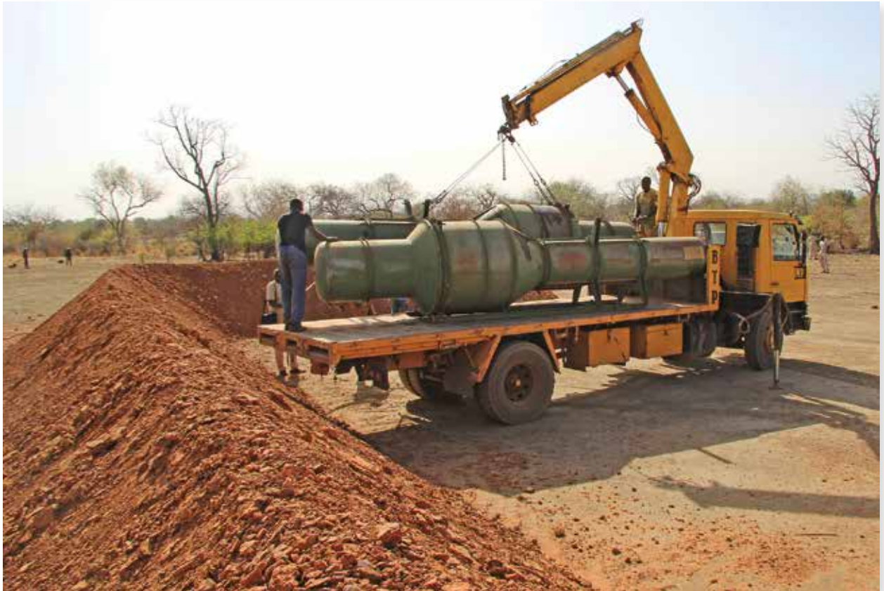
All missiles were moved to the demolition site progressively, with an average of two missiles moved and destroyed every day over two months.
