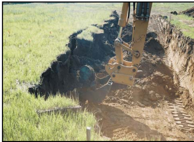
Figure 10. Fracture In Bank
