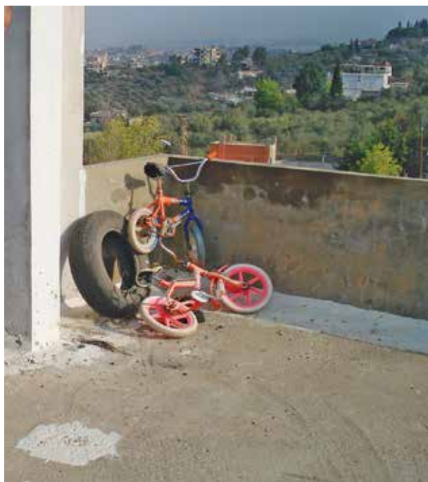
Image 1 (top) and 2 (bottom). Two BLU-63 submunition impact patterns on a roof in southern Lebanon from the 2006 conflict. Note the relatively even distribution of scarring from the fragmentation on the concrete.
