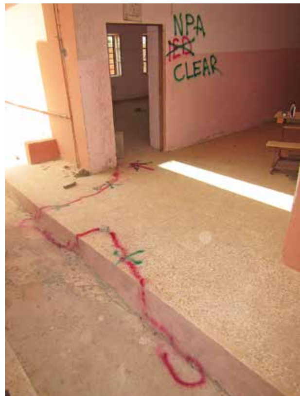
This primary school classroom bears the marking from the HRS clearance process.
