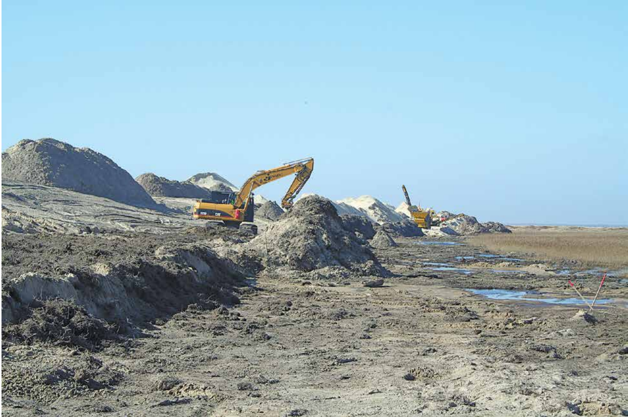
Image 1. The need for remediation after clearance is evident from the Skallingen project. Image courtesy of Martin Jebens and the Danish Coastal Authority.
