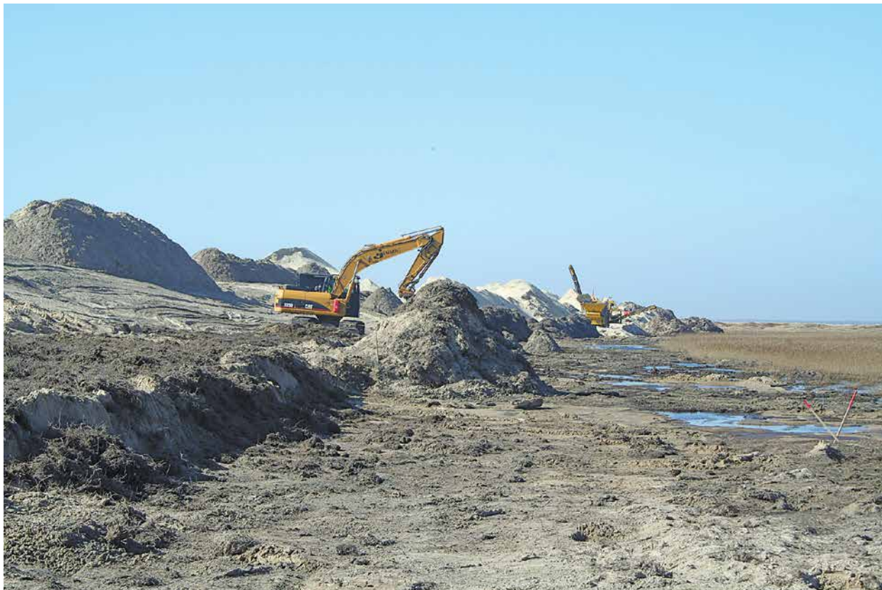
Image 1. The need for remediation after clearance is evident from the Skallingen project. Image courtesy of Martin Jebens and the Danish Coastal Authority.
