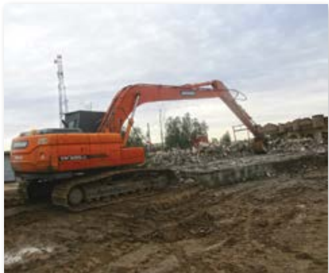
Armored excavator from FSD’s mechanical clearance team in Iraq removing rubble so that villagers can return to their land and rebuild their homes and livelihoods. Image courtesy of FSD.
