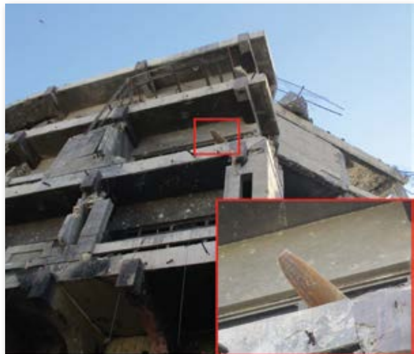
Image 6. A 500 lb. bomb located on the fourth floor of a building with the stairs mostly destroyed, West Mosul, Iraq.
