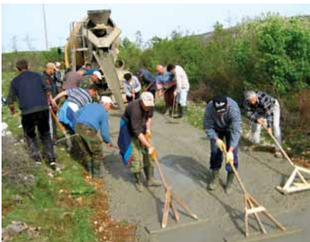
Mine-affected inhabitants actively involved in reconstructing the existing road leading to the community of Burmazi, Bosnia and Herzegovina.
