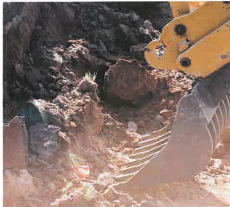
Wall collapses revealing AT mine.
